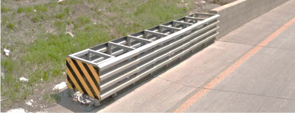
Figure 22. Typical SCI Crash Cushion System (Google, 2016)
